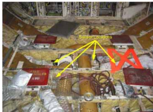
Figure 12. Bay with insulation and ductwork after sensor installation (taped orange X is where several sensors are located)
