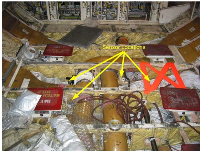
Figure 5. Bay with insulation and ductwork after sensor installation (taped orange X is where several sensors are located).
